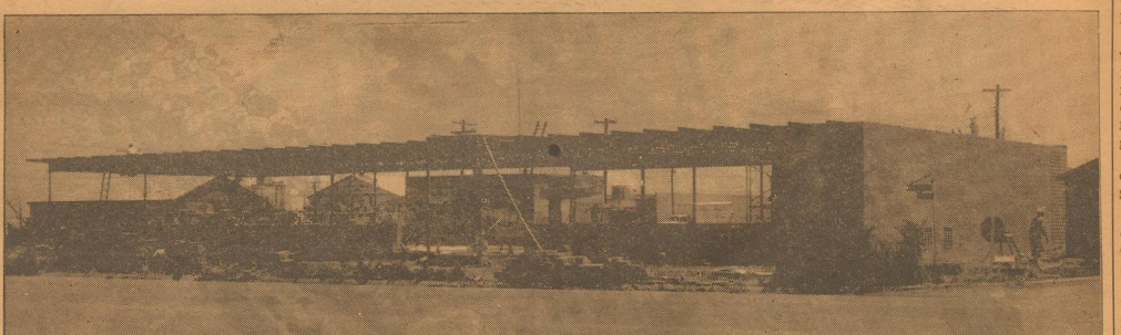
GOING UP —One of the big reasons for Dimmitt's high construction figure for the first six months of 1958 is this new First State Bank building on Bedford Avenue. Costing some $113,000, the new bank will be one of the finest in this area. Killingsworth Construction Company is the builder.
