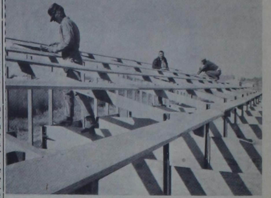
DIMMITT YOUNG FARMERS pitched in Saturday to help the high school FFA boys with their swine and lamb feeding barns south of the city limits. From left, Glenn Odom, Howard Smithson and Ben Holcomb put up framework for the feeder barn's sloped roof. FFA boys inside the city will feed out their project animals here when the barns are completed.
