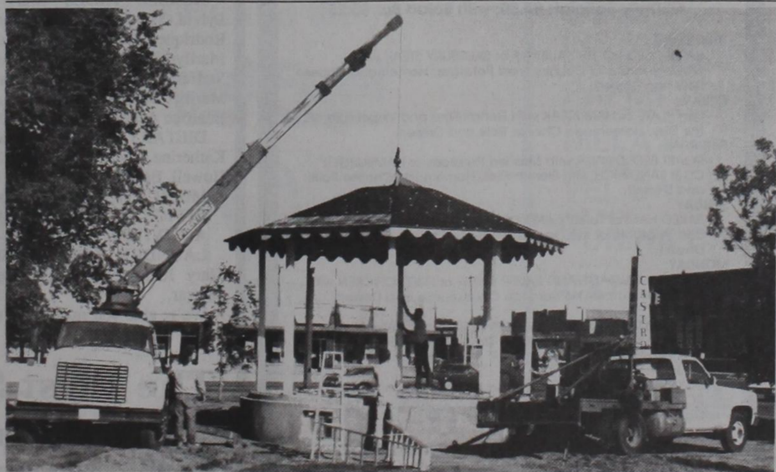
RAISING THE ROOF — Construction work continues on the Centennial Plaza and Gazebo project on the courthouse square in Dimmitt Wed-
