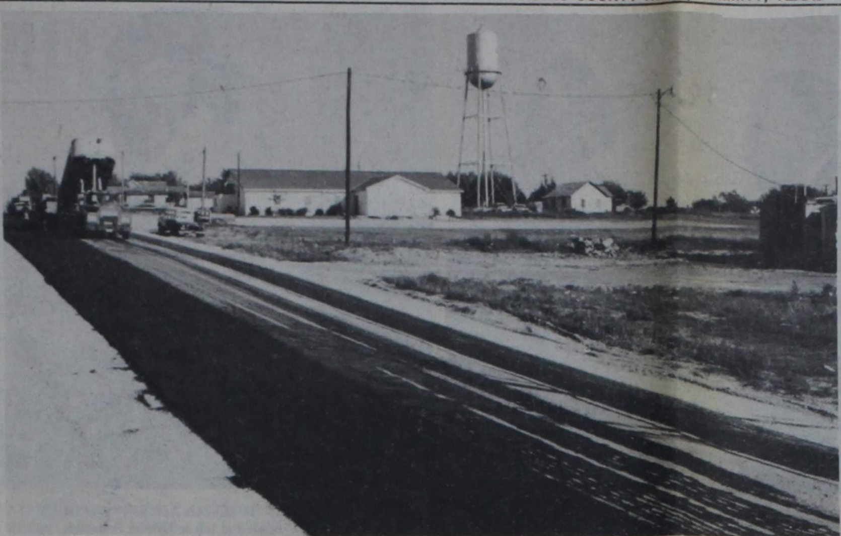
NAZARETH STREETS received more than 2,000 feet of sealcoat last week when the Jake Diehl Dirt & Paving Co. of Hereford applied 1 1/2 inches of hot-mix topping to two east-west streets in a $15,000 project. Here, workers apply topping to the street that runs from the schoolgrounds west past the church and American Legion hall to State 168. Also paved was an east-west residential street on the north edge of the city.
