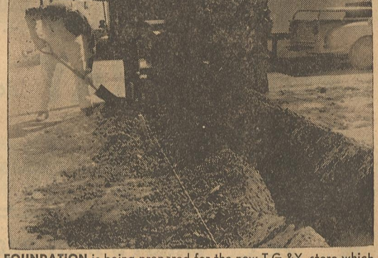
FOUNDATION is being prepared for the new T.G.&Y. store which will be located on Broadway. Ray Lee Construction of Lubbock will build the 6,000 square feet building. Official construction started September 3. Gary Sheppard of Odessa, formerly of Amarillo, will manage the Dimmitt T.G.&Y. store. —Staff Photo
