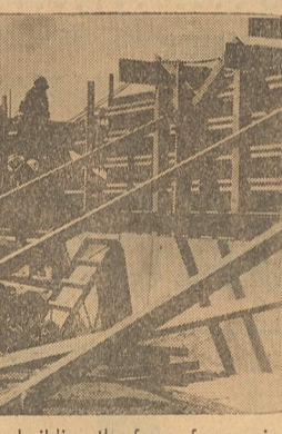
CONSTRUCTION WORKERS are building the forms for pouring cement in the central part of the proposed Western Ammonia Plant. The plant when completed will have a 60 ton per day capacity. Construction should be completed in February, 1964. —Staff Photo
