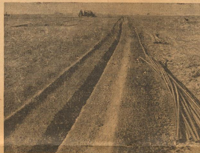
Longer gas pipelines can be installed at a lower cost with Carlon plastic gas pipe. Hundreds of miles of trouble-free pipeline have been installed in Texas High Plains area.
