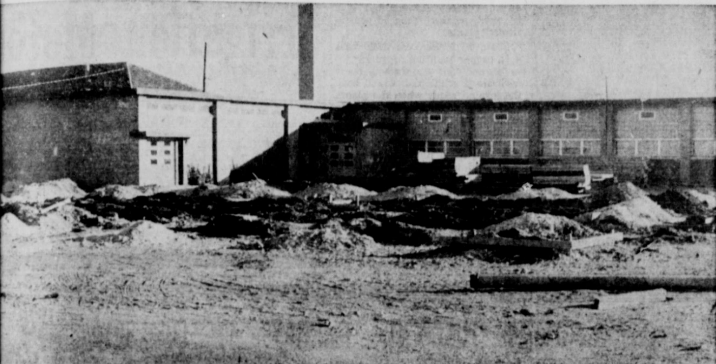
UNDERWAY — Foundation for the new addition to the local school plant is being laid this week, as construction begins for the $2,919 expansion program. The addition shown above will include four classrooms, cafeteria room and kitchen. Other work to be done includes the construction of a woodworking shop building, conversion of the present cafeteria into a library and science laboratory and conversion of the present shop building into a fieldhouse. REVIEW Photo
