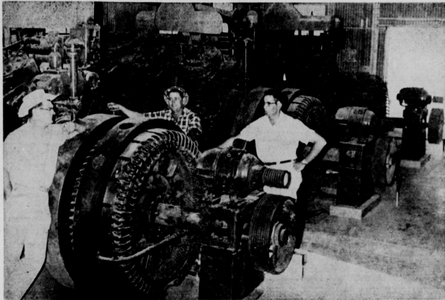
PLAINS POWER PLANT — Here is the three huge units which will supply electric power to Plains in the near future. The equipment is seen during the dismantling being done by Prewitt, Jones and Ballard of Brownfield. After everything is taken apart, there will be a complete rebuilding of the machinery before it is moved to Plains. Not seen is the oil filter, starting motor and auxiliary power unit for the plant. Also included is the building, various tanks and an outside building and cyclone fence. Here with the engine are left to right: Bennie Jones, partner of the company; L. H. Lee, employee of Prewitt, Jones, Ballard and Clyde Amonett who is presently employed by the firm and who has been hired by the city council to operate the plant after it is installed. Mr. Amonett operated the plant in its present location for a number of years.
