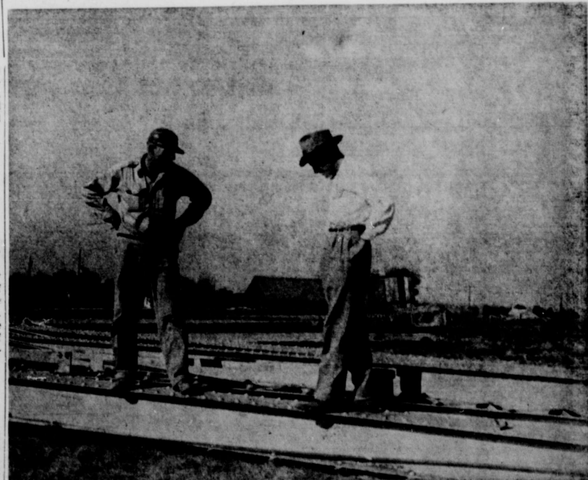
NEW WATER TOWER — City Water Superintendent John Camp, left, and Mayor Roger Curry look over the mass of steel water storage tank which will be put together and erected just west of the present city water tank. The new tank, purchased in Odessa for $18,000, is of 100,000 gallon capacity and is said to be in excellent condition by the city engineer. The tank is a used one and has been sand blasted and completely reworked to give Plains maximum use, according to Mayor Curry. —REVIEW Photo
