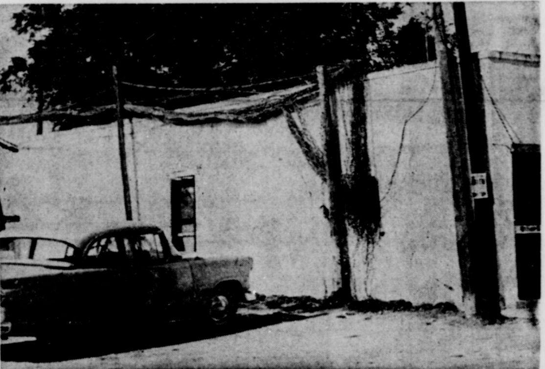
IT'S NOT A VINE — What you see on the side of the telephone company building is not a dead vine, it's a great maze of wires that now will be removed as the Romain Telephone Co. begins modernizing. Work on the new central office building should get underway in the next week or two. After the move the company plans to lease this structure. REVIEW Photo
