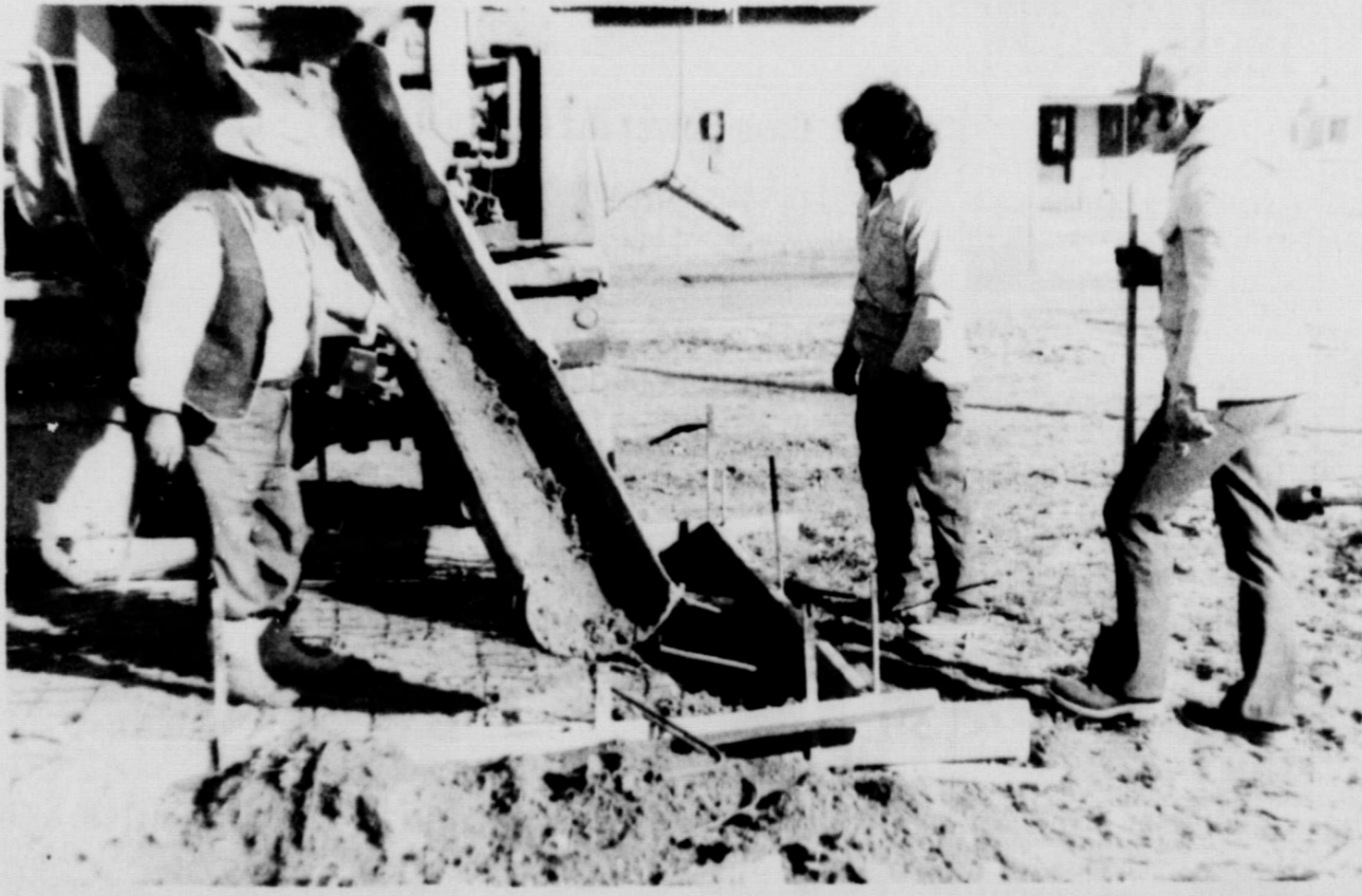
JERRY FORD, far right, watches as cement is poured for the foundation for his equipment building and microwave dish sections of the system by mid-April, with service through the new Lockney cable television system. Ford says if the good weather continues, he may be able to start turning out most of the city planned by mid-May.
