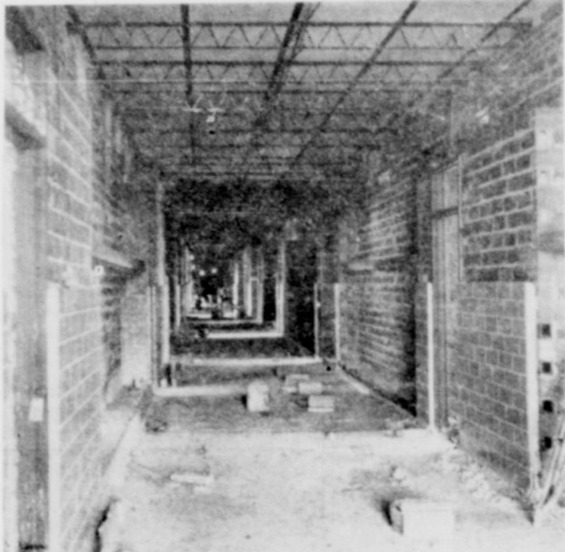
Here is a view of the long hall which connects the classrooms, the gymnasium, rest rooms, cafeteria and administrative offices in the new building to the old building. The tile wainscoting just beginning here is now complete through the entire hall but the plastering above the wainscoting is yet to be done.
