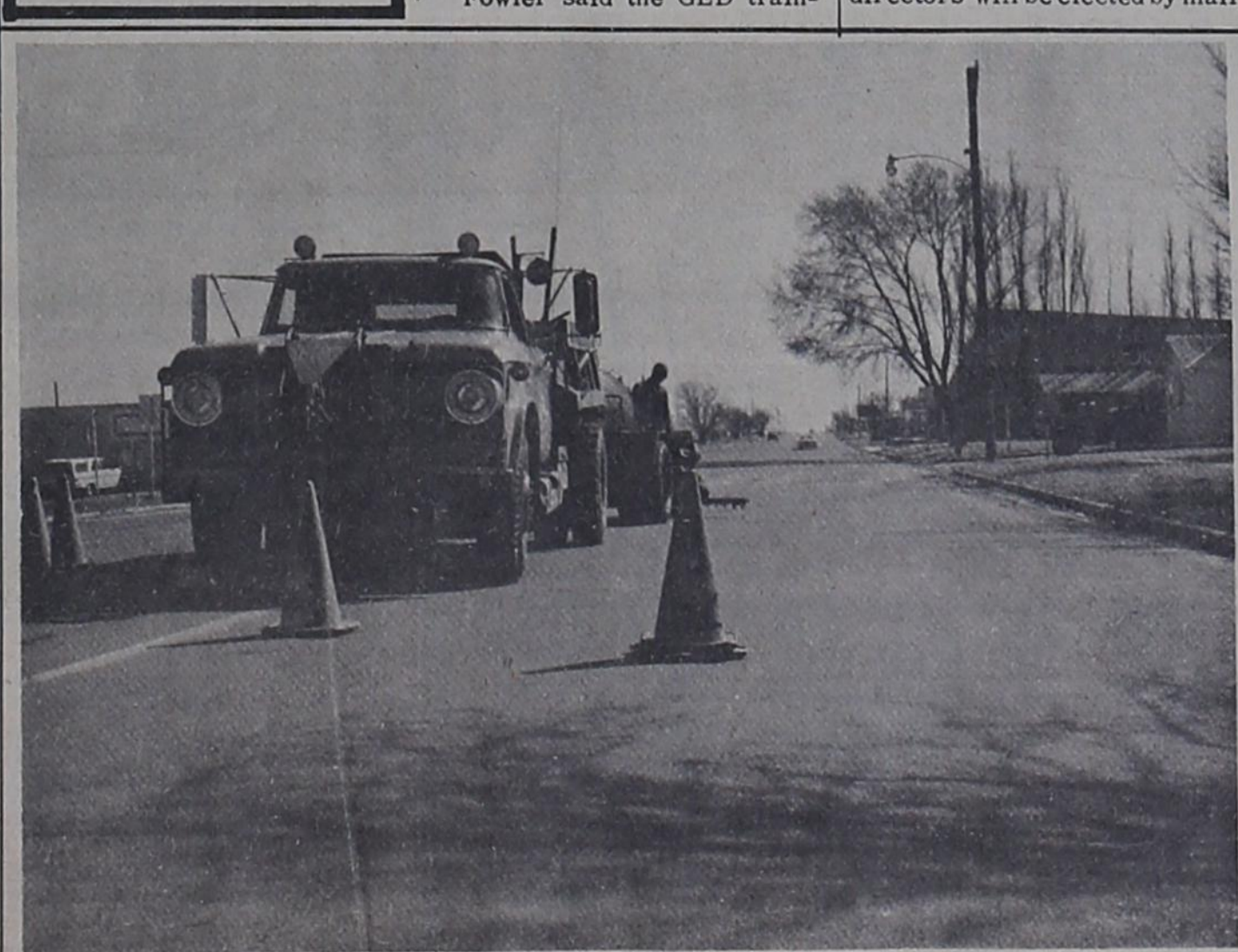
REPAIRS --- State Highway Department crews this week are repairing FM 1731, Third Street in Bovina and other state roads, as a result of damage received during the snow and ice that remained on roads during late December and early January. Damaged areas were filled in, then received a new asphalt and gravel job.
