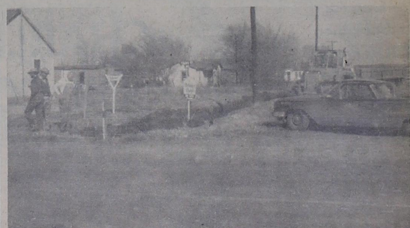
DRAINAGE IMPROVEMENTS--State Highway Department crew has been improving Third Street water drainage situation during past few days. Here, a ditch off Third Street is being deepened. Shown at left are Tom Paine, Highway Department Foreman Lloyd Killough and E. H. Young, who lives in house at left. Completion of the work will allow water to drain from ditches on Third faster.
