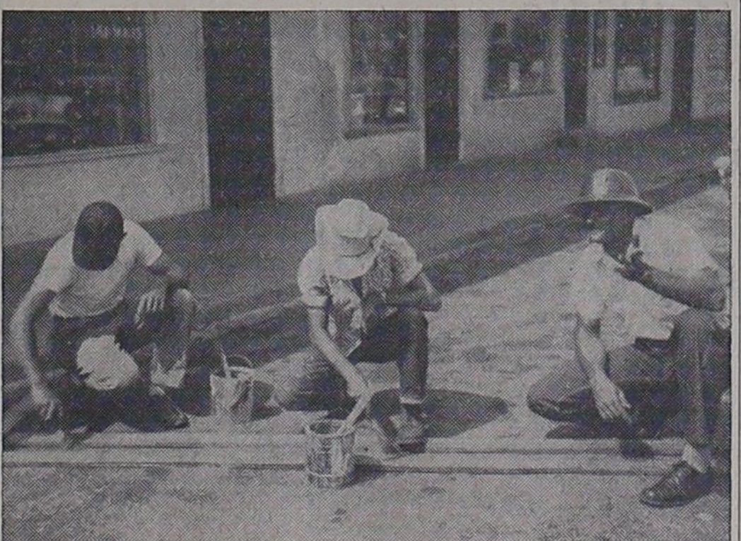
STREET PAINTING—Painting of designated parking space on North Street was being done the first part of the week. One purpose of the painting is to cut down on the amount of vehicles that park in the middle of the street. Henry Minter, right, city water superintendent, is in charge of the painting. The painters pictured are James Wade, left, and Bill Pruitt.
