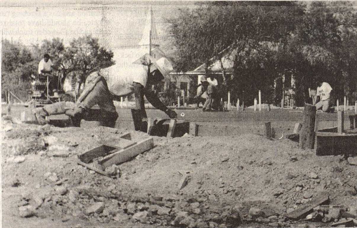
Construction crews finish pouring the slab for Brackett ISD's new academic wing. The workers began the project at 3 a.m. last Thursday. Superintendent Taylor Stephenson said it took an estimated 350 to 400 yards of cement to complete the slab. The framing for the building will be steel in a prefabricated frame that is expected to be put in this week. Brackett News Photo by J.J. Guidry
