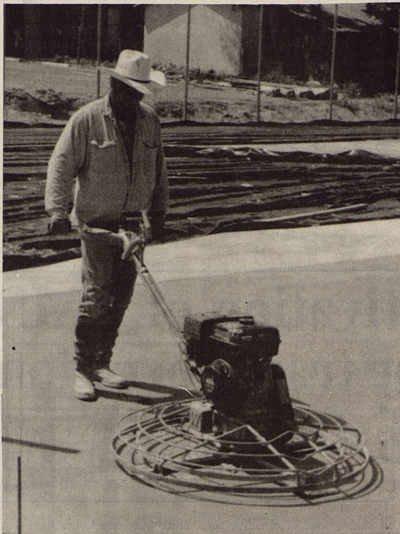
Sam Carter of San Angelo spreads concrete at Brackett ISD's new tennis complex. Brackett News Photo by J.J. Guidry
