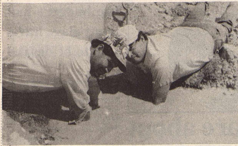
City of Brackettville employees Richard Ortega, left, and Domingo Villarreal were literally up to their shoulders in work last week. A three-fourths inch water pipe broke outside of the Kinney County Appraisal District building. The cause of the breakage was time and a rusty pipe. Brackett News Photo by Margie Allen
