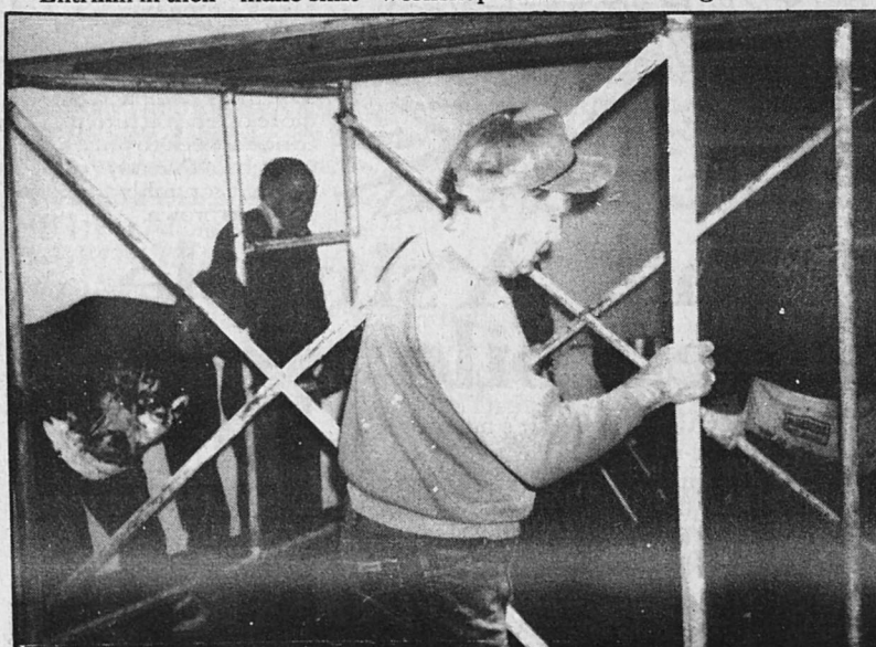
From left, Peter Pohl and Warren Outlaw get assistance from Newell Mayberry and Ray Entrikin in moving a scaffold that Outlaw used to stand on and install ceiling fans.
