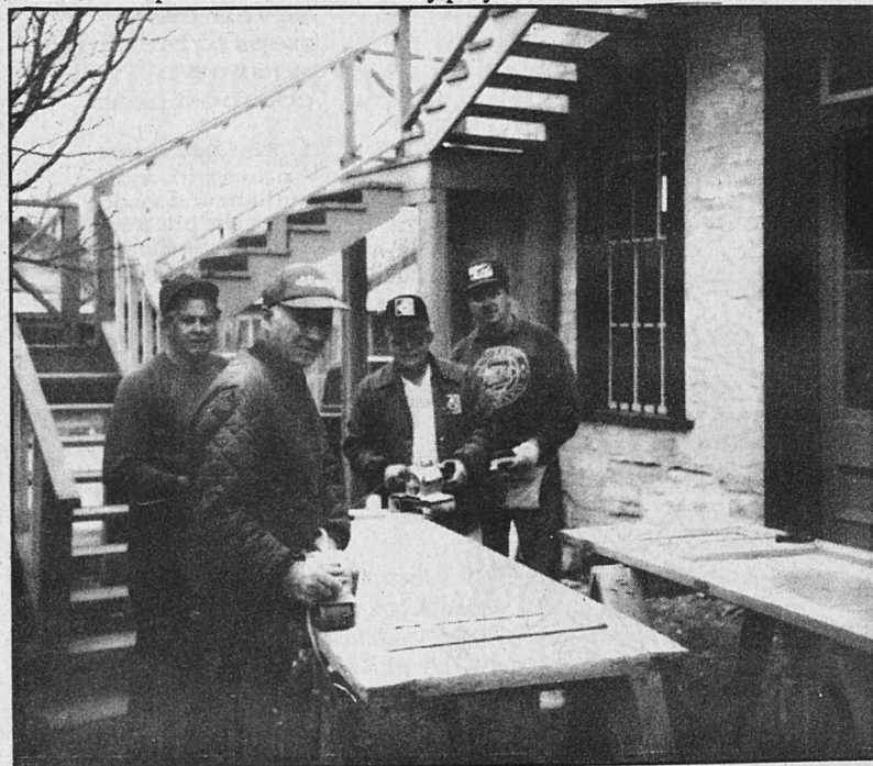
Woodwork was repaired and refinished as evidenced in this picture showing, from left, Newell Mayberry, Jake Zell, Cecil Apperson, and Ray Entrikin in their "make shift" workshop behind the building.
