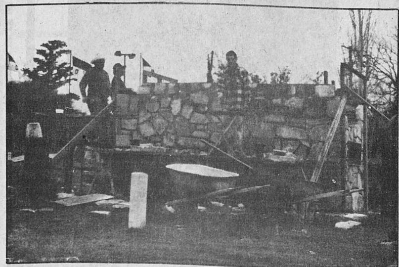
The rock base of the "Empty Saddle" statue has been rebuilt. The horse is undergoing some repair work and will soon be returned to guard duty at the Fort Clark entrance.
