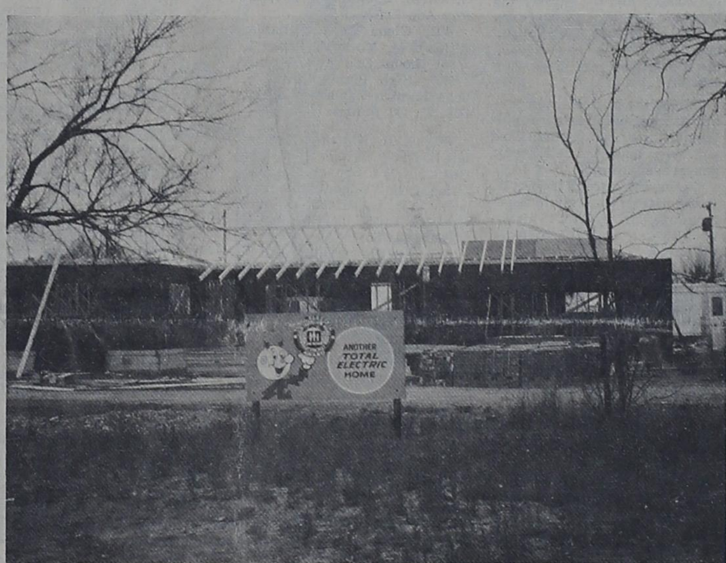
HOME CONSTRUCTION --- One of several new houses under construction in Bovina is this one, being built by Mr. and Mrs. Dudley Hughes. It is located on Highway 86, just west of the Third Street intersection. Plans are presently being made to build several new homes in Bovina's Ridgelea, according to A. L. Glasscock, developer.
