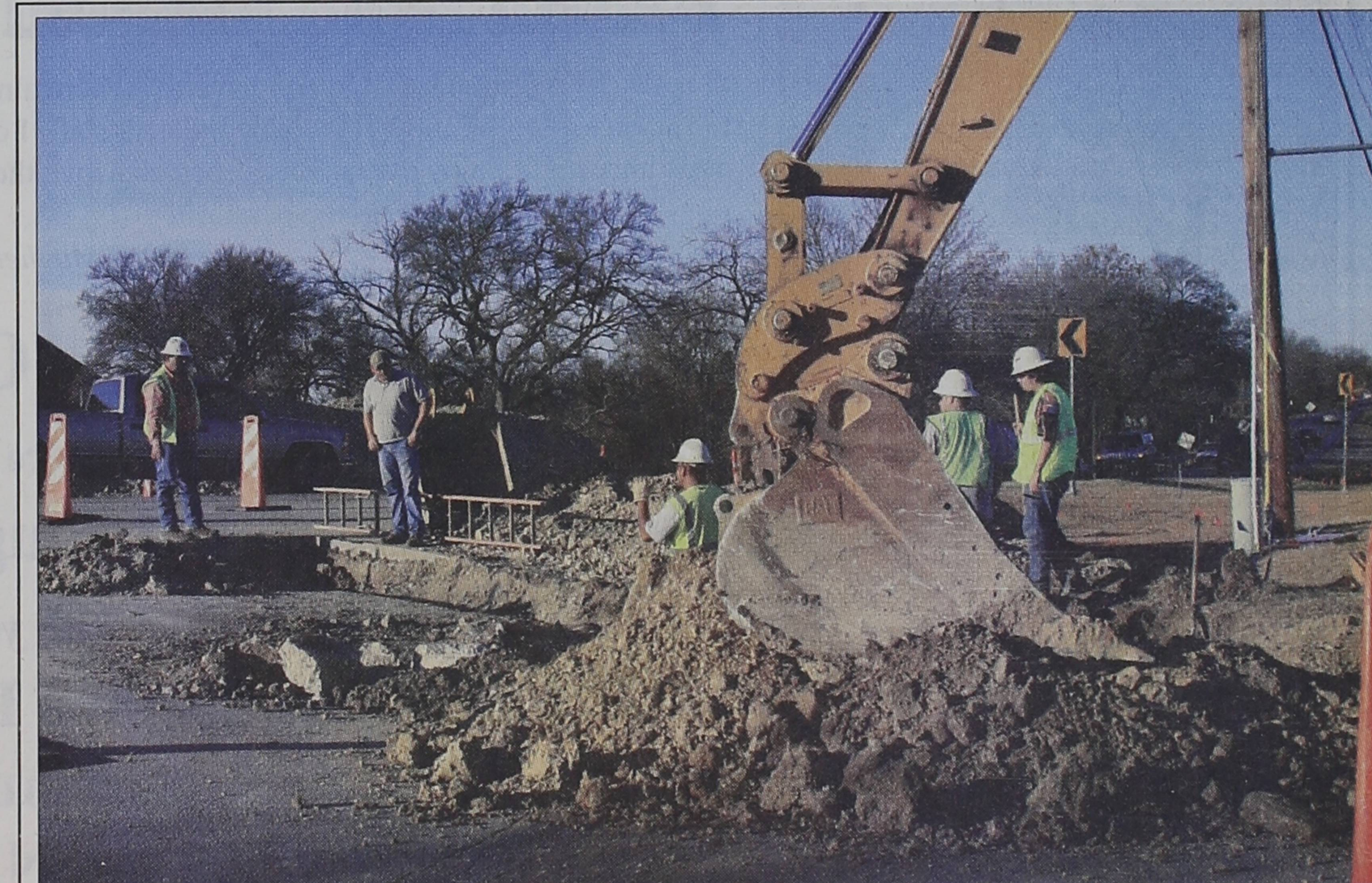
Manuel DelaGarza (left) of Larrett, Inc. discusses construction work with John Cranson of the City of Rockwall Engineering Department about boring under Highway 740 (Ridge Road) for a water line at the intersection of White Road. The project is expected to take five months and is part of preparations for the state's work on FM-740 construction project. Staff photo by Tim Burnett
