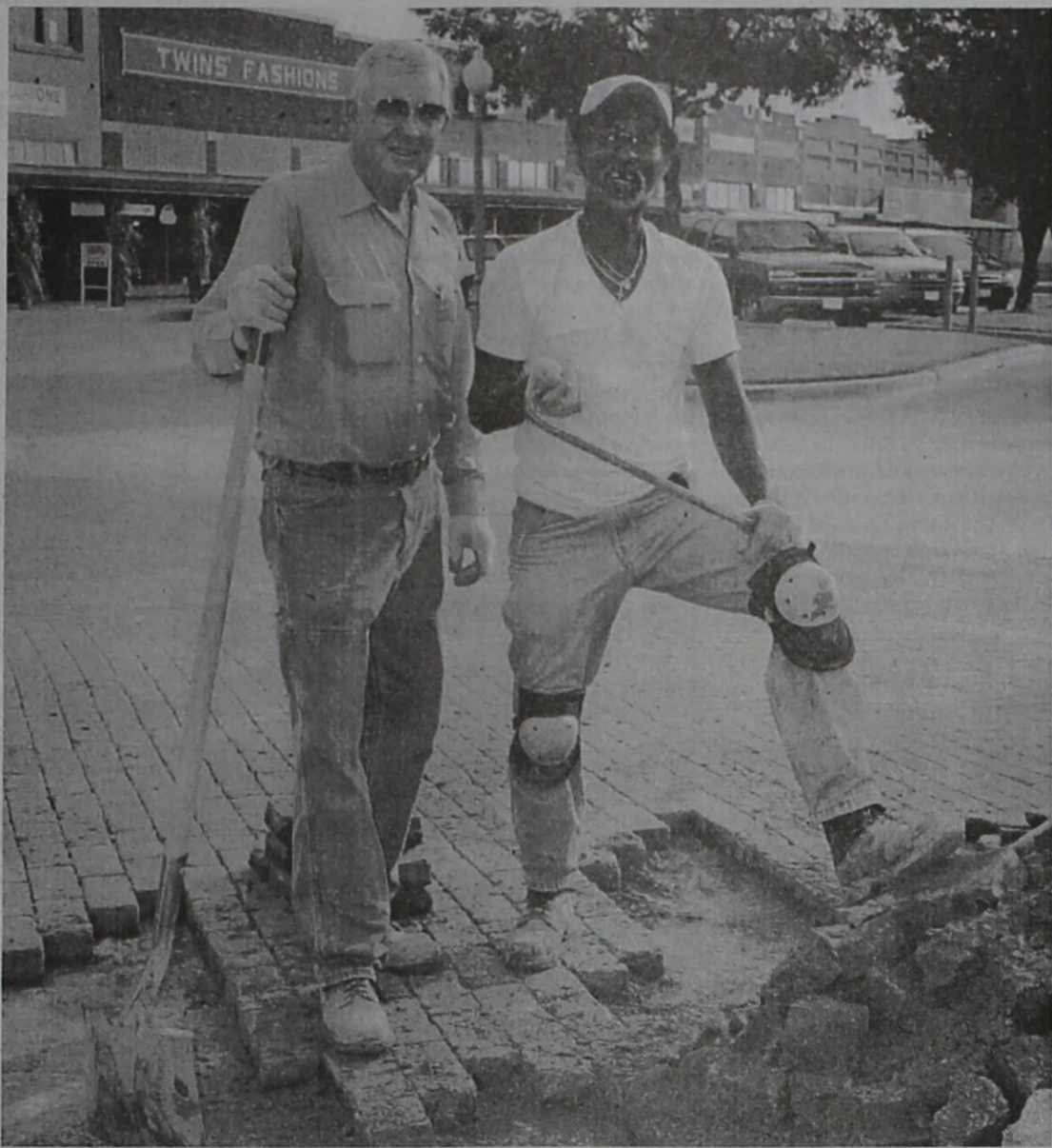
Bo Jackson (left) and Johnny Jefferson are replacing bricks on Main Street.
