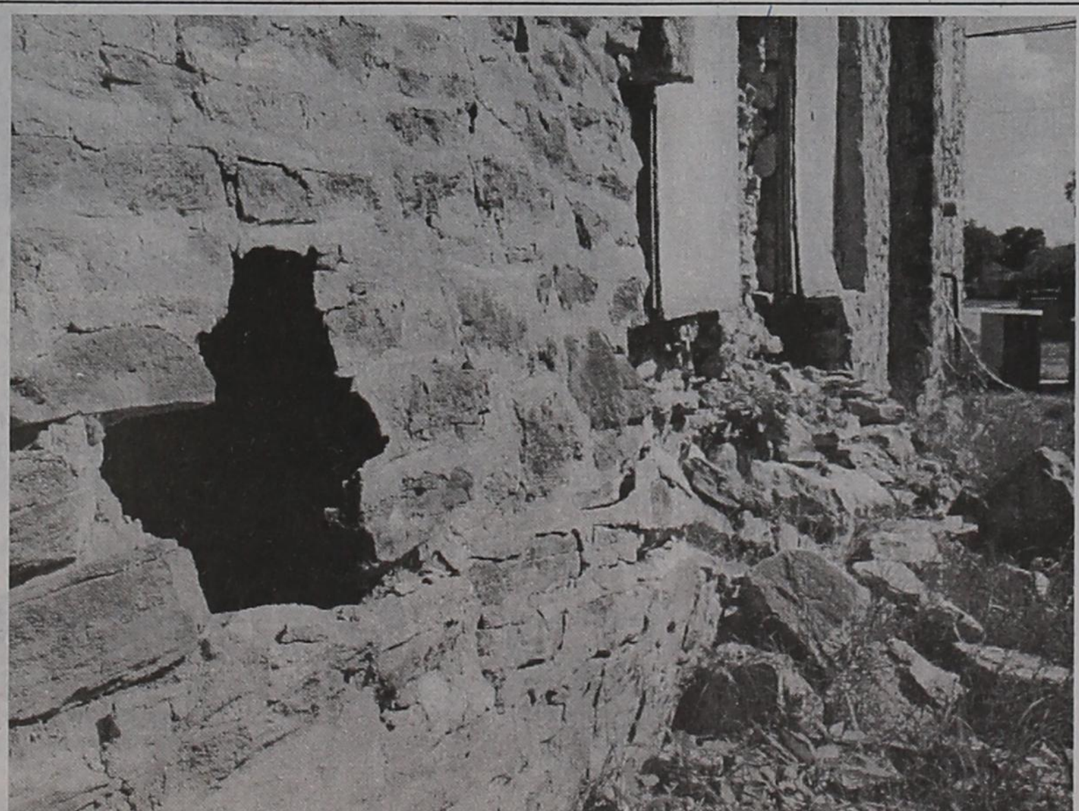
The sand stone outer walls of the historic Algerita Hotel building on East Main Street demonstrates the difficulties facing restoration planners. (Photo by Tim Burnett)
