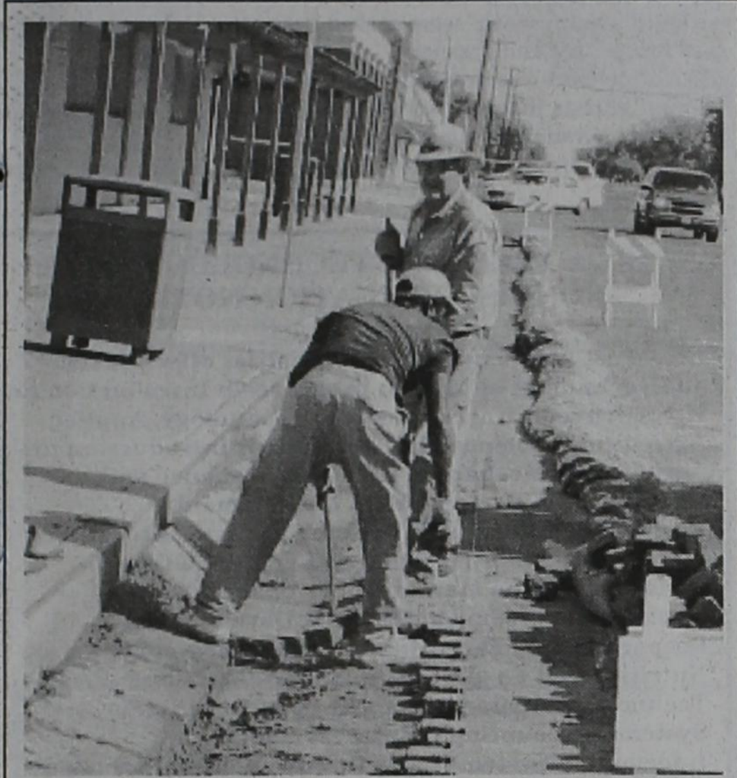
Bo Jackson (back) is leading the crew repairing water damage to the historic downtown street adjacent to the Algerita building. A new drain will be constructed to keep water from further damaging the bricks.
