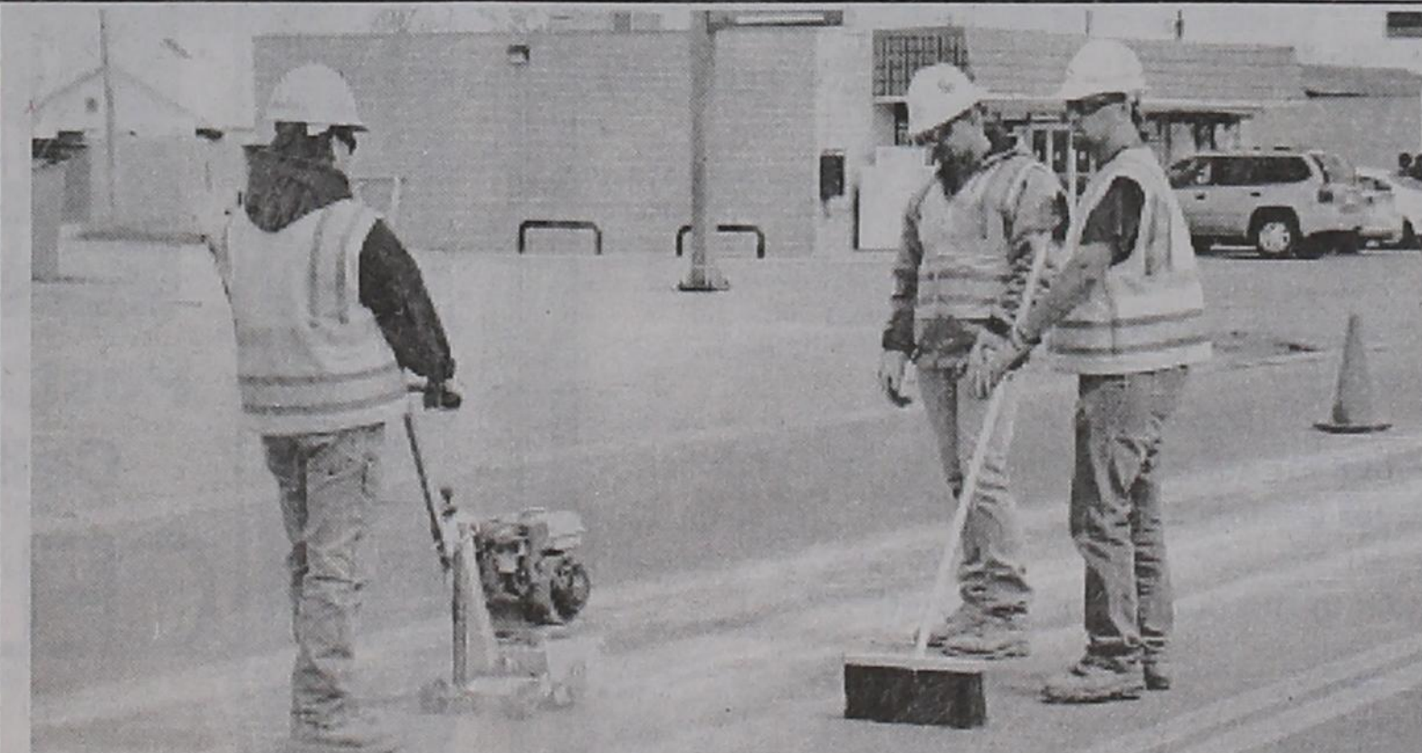
Texas Department of Transportation crews were busy recently removing the old striping on U.S. Hwy 380 adjacent to the middle and elementary schools. Scraping off the old paint were (left to right) Larry Valdez, Robby Dean and Richard Martin. The striping returns the roadway to its traditional two-lane status, removing the turning lane which had been requested by the City of Post and Garza County Sheriff's Department.
