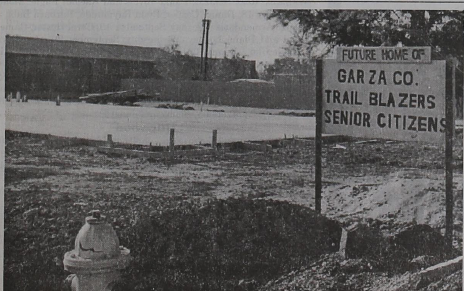
Construction work is proceeding on the new senior citizen facility, located at the corner of Avenue I and 10th Street. The Trailblazers continue to seek financial assistance with necessary interior materials. (Photo by Thomas Zachary)
