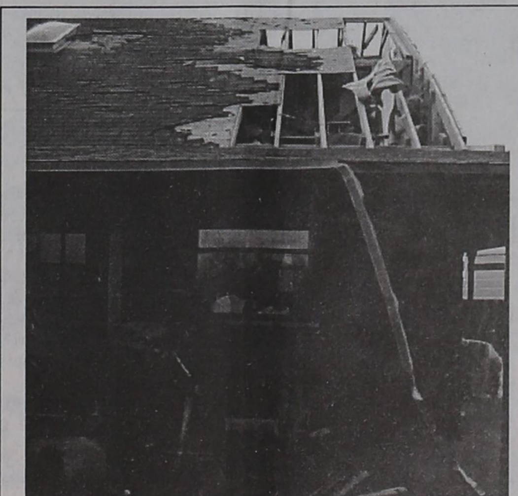
Dan and Jennifer Fumagalli's home suffered extensive damage from last Sunday evening's tornado that ripped through Garza County. (Photo courtesy Dan Fumagalli)
