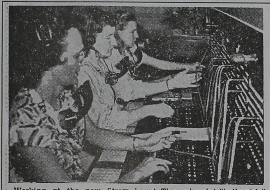
Working at the new Stromberg-Carlson Switchboard in the local Southwestern Associated Telephone office are, left to right, Jewell Parsons, Theda Jo Bilberry and Virginia Sturdivant. These cheerful "hello girls" give excellent service to their telephone customers and add free information on everything from "where the fire?" to "what time is it?"
