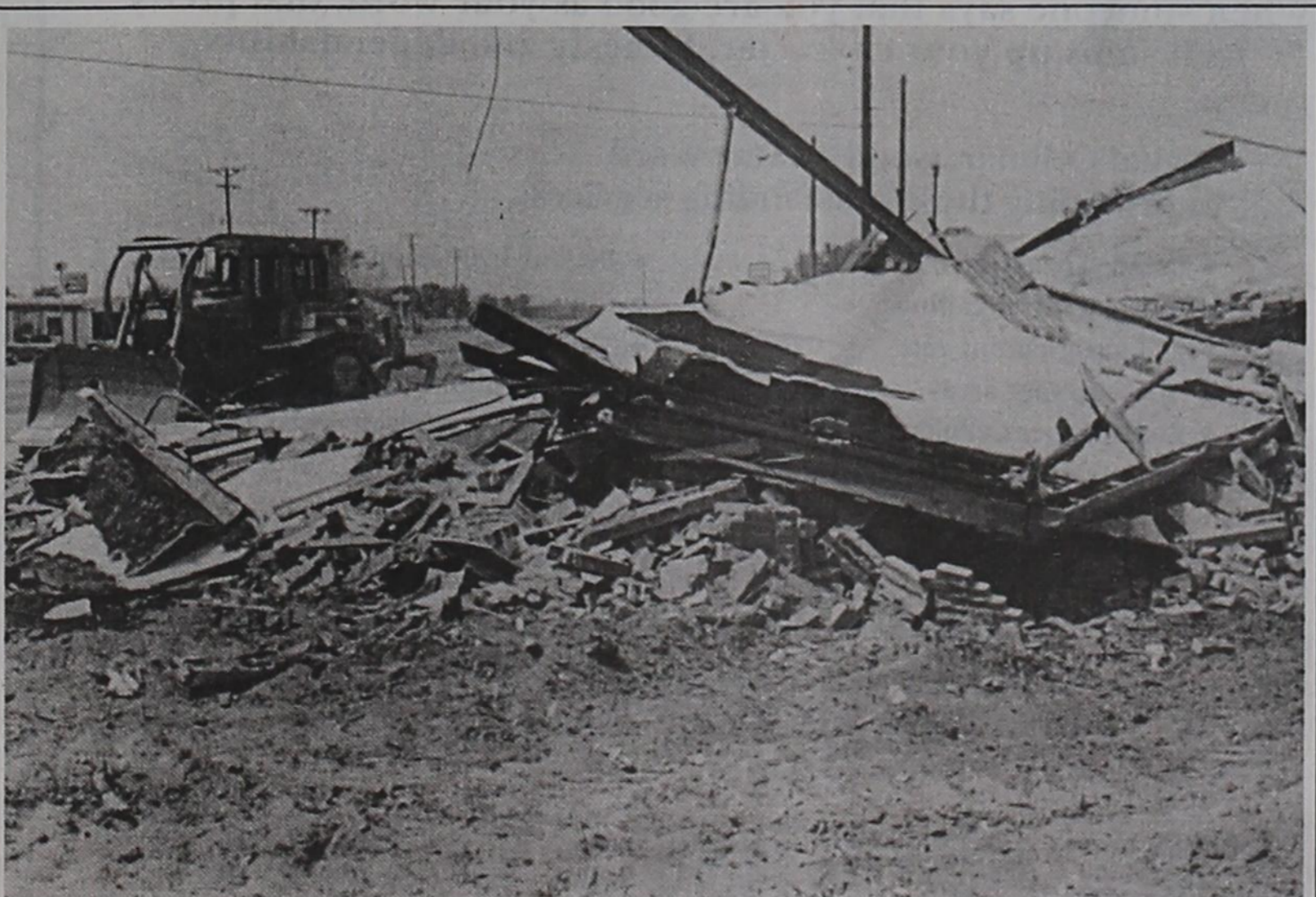
The old Shamrock station at the corner of 15th and Broadway (U.S. Hwy 84) was demolished last week, making room for a new business in Post. The Lubbock office of Subway told The Post Dispatch this week that construction will start in the next few days, with a July 1 opening date.
