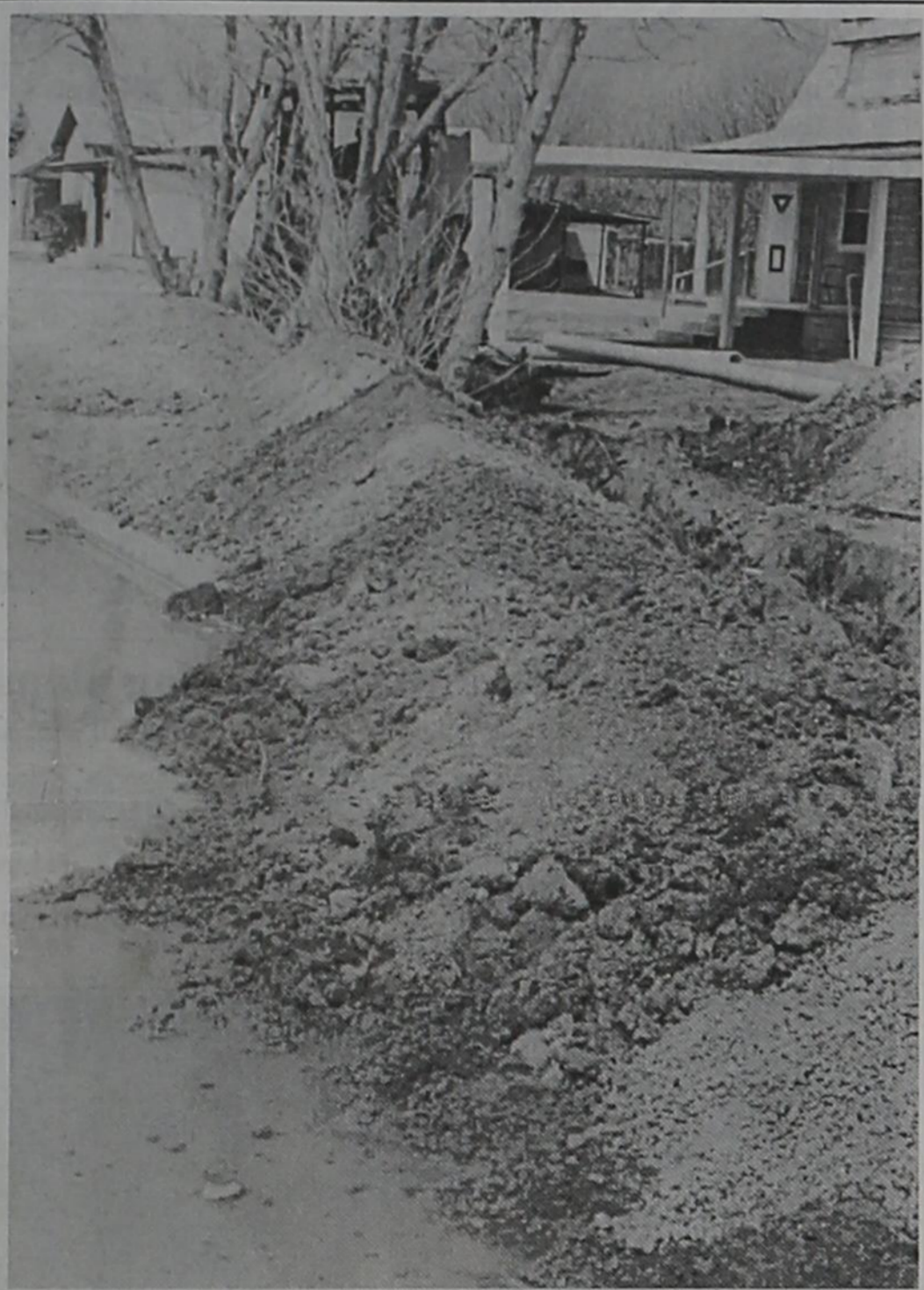
Water line replacement in Post is proceeding, with some disruption to traffic in various neighborhoods. Construction crews are replacing old lines as part of the city's continuing efforts at improving the water system.
