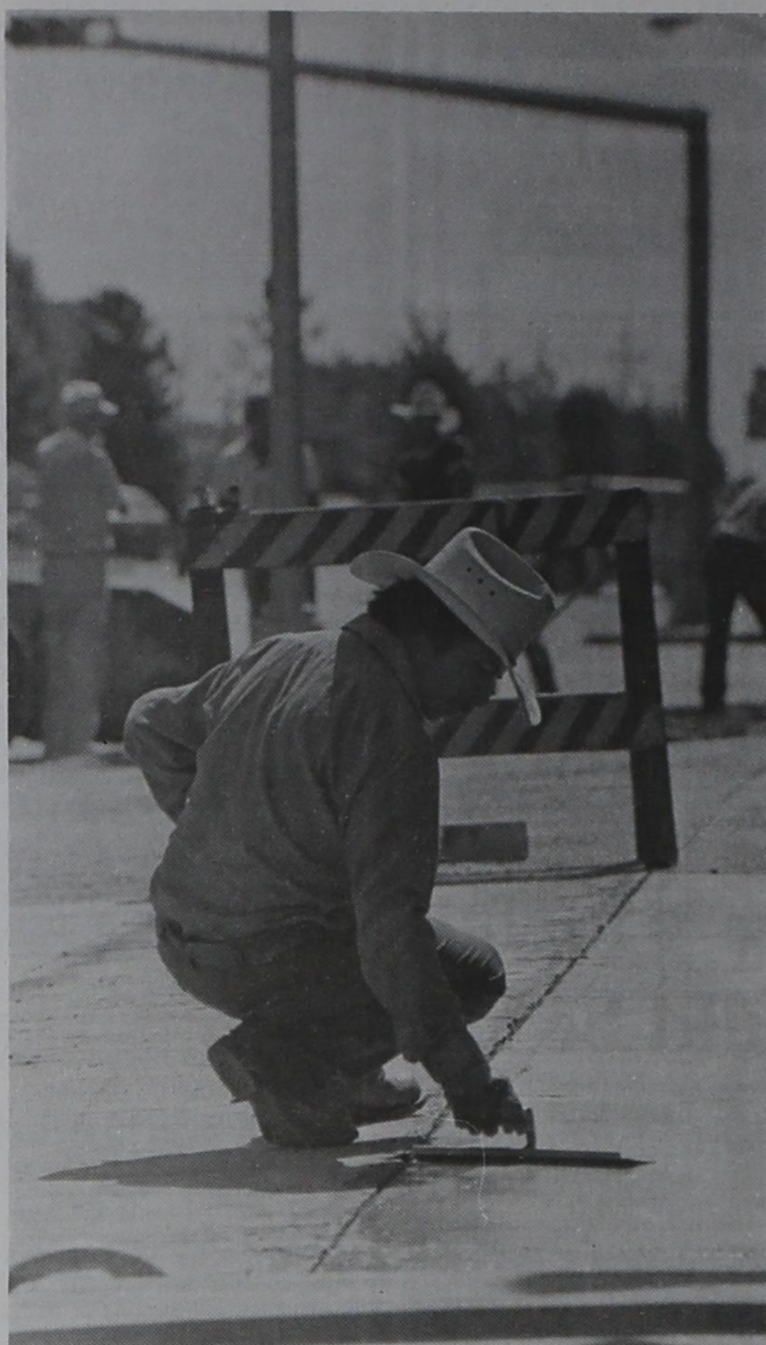
Benjamin Casillas puts the finishing touches on new concrete for the sidewalk in front of Fashion Cleaners. Working on a contract with the city, Bo Jackson and his crew completed the work last week. Business owners and the city share the cost of the work based on ownership of the sidewalk. (Photo by Tim Burnett)
