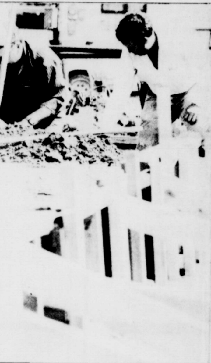
Plumbers install water and sewer lines as preparations for the foundation of the new City Hall began here this week. The foundation was expected to be poured by the end of the week. (Staff photo)
