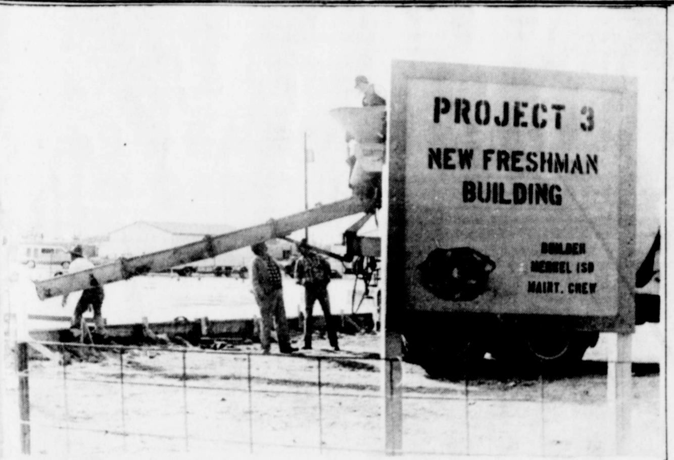
§ The slab for the new Freshman Wing at Merkel High was poured Friday. The project should be completed by June 30th and MISD maintenance crews will be doing most of the construction. [Staff photo]
