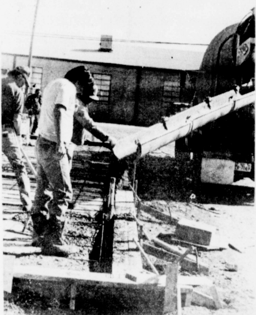
More than 30 trucks of cement planned to be completed in June were used in the slab for the funding is from surplus MIS Merkel High Freshman Wing. The 11,800 square foot building is (Staff photo)
