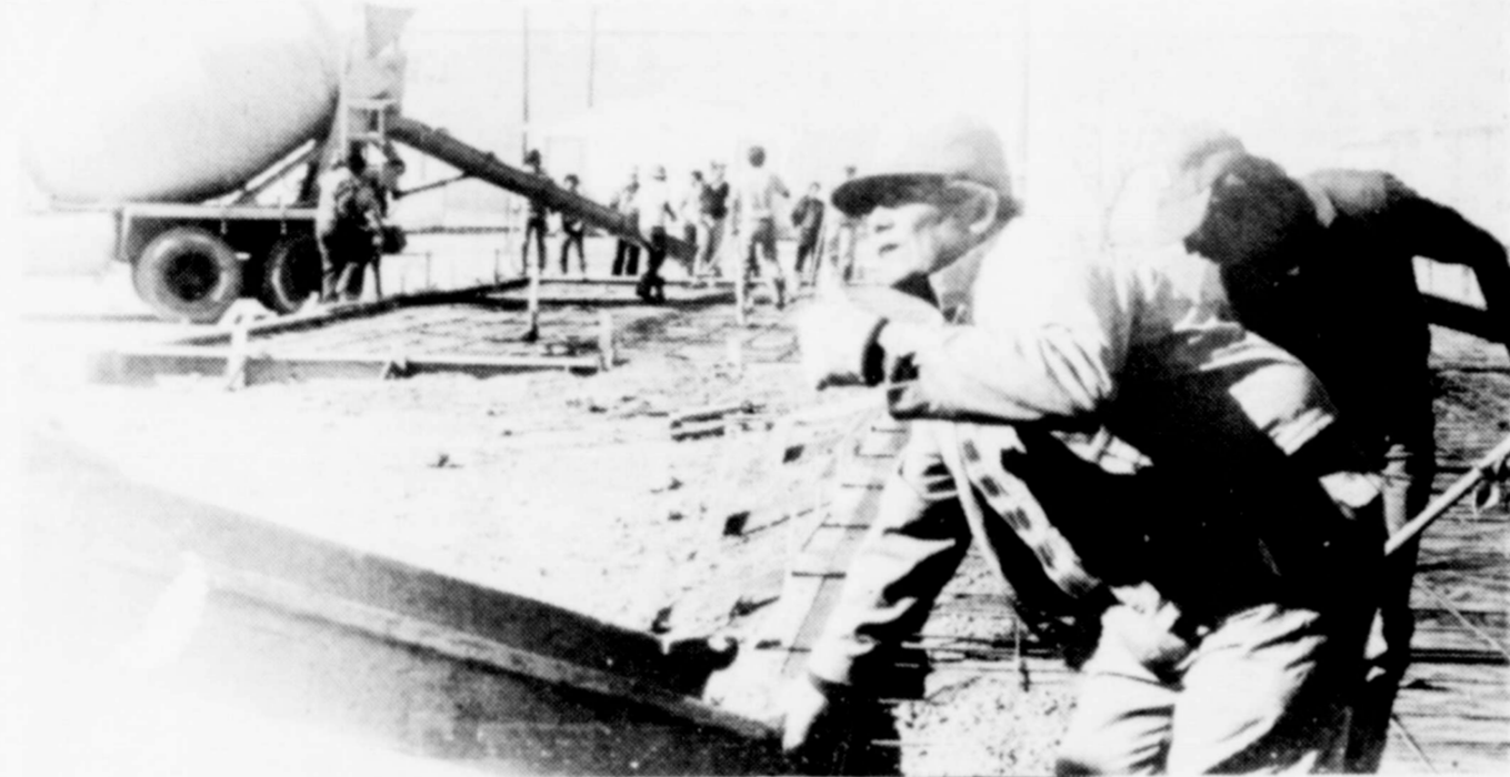
A concrete workers asks for more concrete at the new Freshman Building at Merkel High. The
