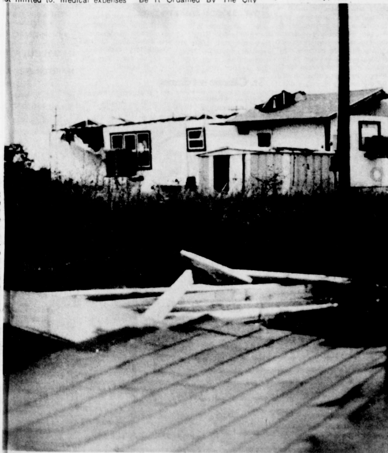
§ A tornado ripped the roof off a trailer house owned by the Harris family a mile southeast of Merkel. The roof had just been recently completed after a twister in May
