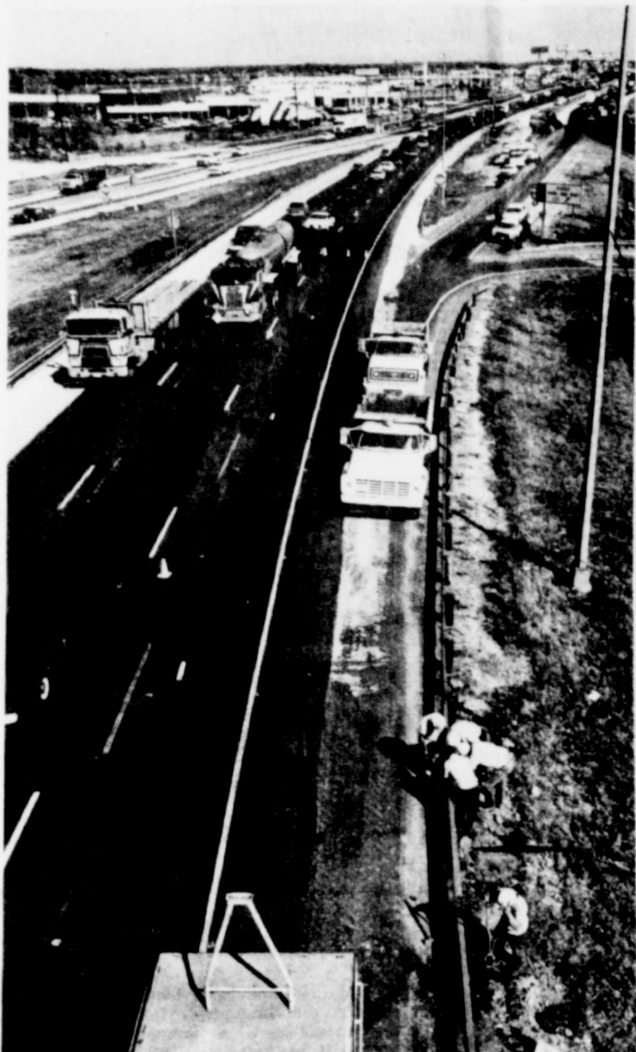
These highway workers stake their lives on the skills of 50,000 drivers during one day of maintenance work on freeway guardrails.
