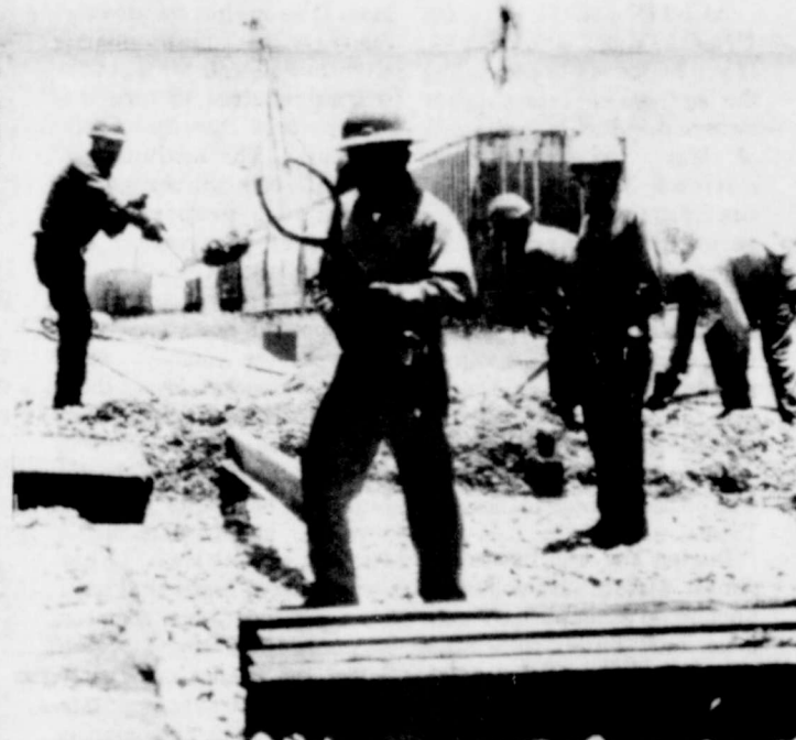
Missouri-Pacific employees lay down new ties at the Oak Street crossing last week. The railroad also put a new drainage system under the crossing. (Staff photo)
