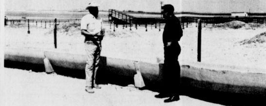
CONSTRUCTION SITE -- Bob Bliss and Max King are shown near the feed troughs being built of concrete for the new feed lot under construction. Loading chutes can be seen in the background.
