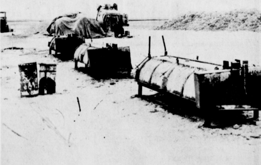
IN FORMS -- These are the concrete feeding troughs being built for the new King Feed Lot. Three of them are pictured in the foreground after being poured from the large mixer.
