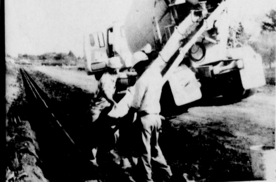
CONCRETE POURED AT SCHOOL —This curb at the school campus in Crowell. The curb is part of an RC&D project to beautify the local campus. The project is funded by the local school and RC&D money.
