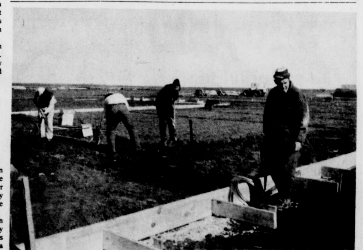
FOUNDATION WORK AT BAPTIST CHURCH —Al Sibert, right, along with other workmen, are pictured above as they prepare the groundwork for the foundation of the new
