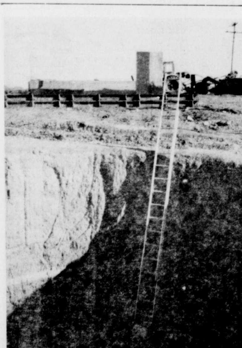
WORK ON NEW CITY DISPOSAL SYSTEM—In the picture above is shown a portion of the work being done at the City of Crowell's new disposal plant. The ladder in the above picture vividly shows the depth of the hole which is being lined with concrete. In the background is framework for more concrete pourings. Chatfield Construction Co. is building the new system.
