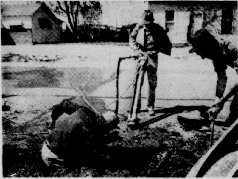
REPAIR WATER MAIN BREAK —These three City of Crowell employees were busy Sunday morning repairing a break in a water main on North Main Street. R. L. Woodard, left, and Melvin Dishman, right, are shown digging as Milton Hunter (center) operates a portable pump taking water out of the work area.
