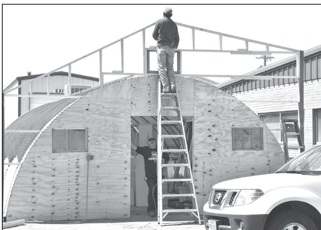
Lots of work going on in and around Friona these days. Top photo: Parmer County Implement is nearing completion on its addition. Middle photo: The new Family Dollar store is taking shape. Bottom photo: Misty Frye is renovating her greenhouse.
