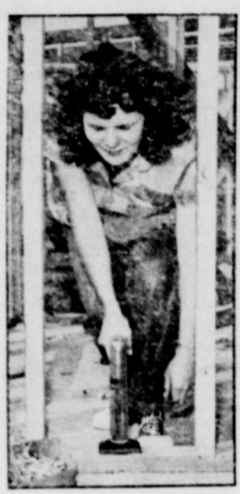
THE NEW "400" — It's the "Blue Overalls," not the "Blue Book" for Mrs. Martha Schubert, of Los Angeles, Calif. She is one of 400 union card-carrying women carpenters in the Los Angeles area. She uses a gunpowder-powered device to fire three-inch steel pins that attach wooden framing to concrete flooring of new homes.
