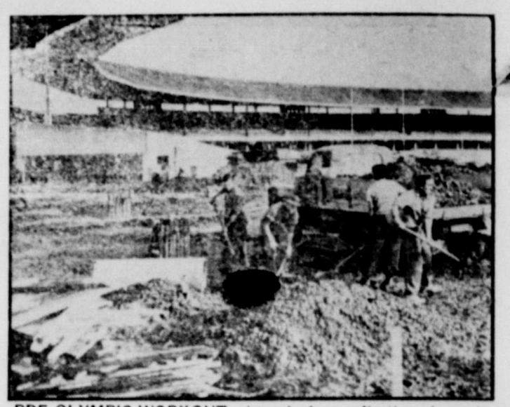
PRE-OLYMPIC WORKOUT —A workaday application of muscle skill is displayed at Melbourne, Australia, where workmen demolish portion of a stadium grandstand at Melbourne Cricket Ground in preparation for the 1956 Olympic Games. New grandstand will seat 43,000 and total spectator capacity of the grounds will be 104,000.
