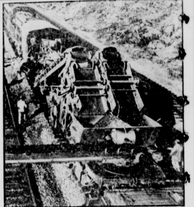
VACUUMING THE TRACKS —This complex contraption is a railroad sweeper. It's used to clean and refurbish the roadbed. The oversized vacuum, which travels on a flatcar, carries off dirt and waste materials on the conveyor belt at the rear.
