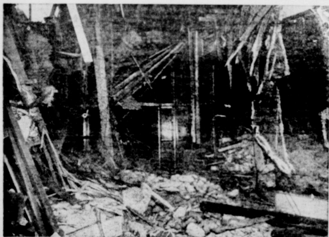
SHOPPERS TRAPPED AND KILLED . . . Two persons were killed and many others were trapped by falling beams and ceiling when the roof of this building, a Lerner's clothing store, collapsed. The tragedy took place during the violent earthquakes that rocked Bakersfield, Calif. The building is typical of the damage done to stores in the downtown area of the California city. However, other shoppers in the downtown area were fortunate that some of the roofs resisted the quake and remained secure, as it was this type of damage that caused most of the deaths reported after the Bakersfield quakes. Scientists foresee a year more of California quakes.
