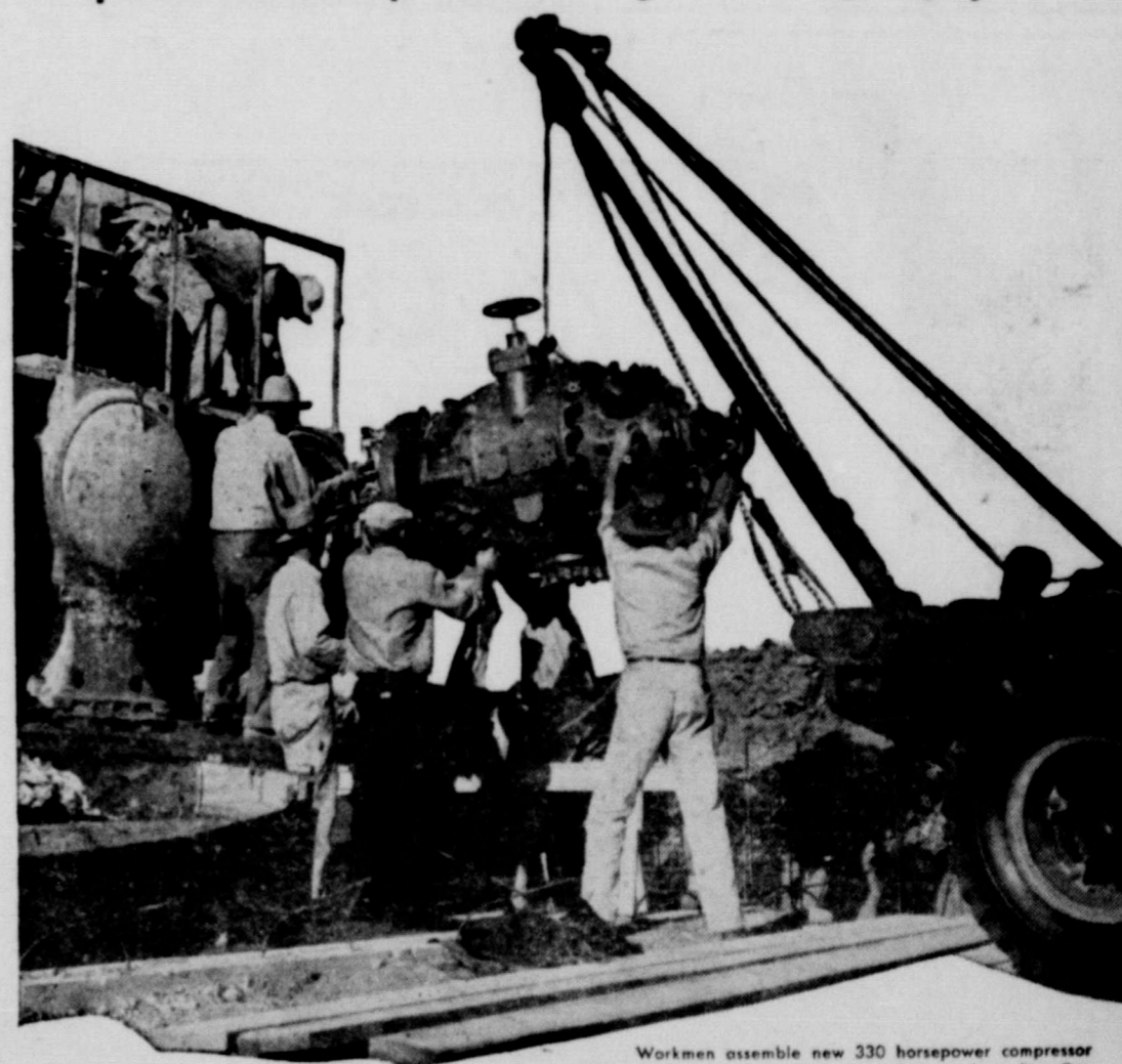
Workmen assemble new 330 horsepower compressor engine at one of six new stations on Lone Star Gas System. Engines totaling 9,640 horsepower were added in recent months.
