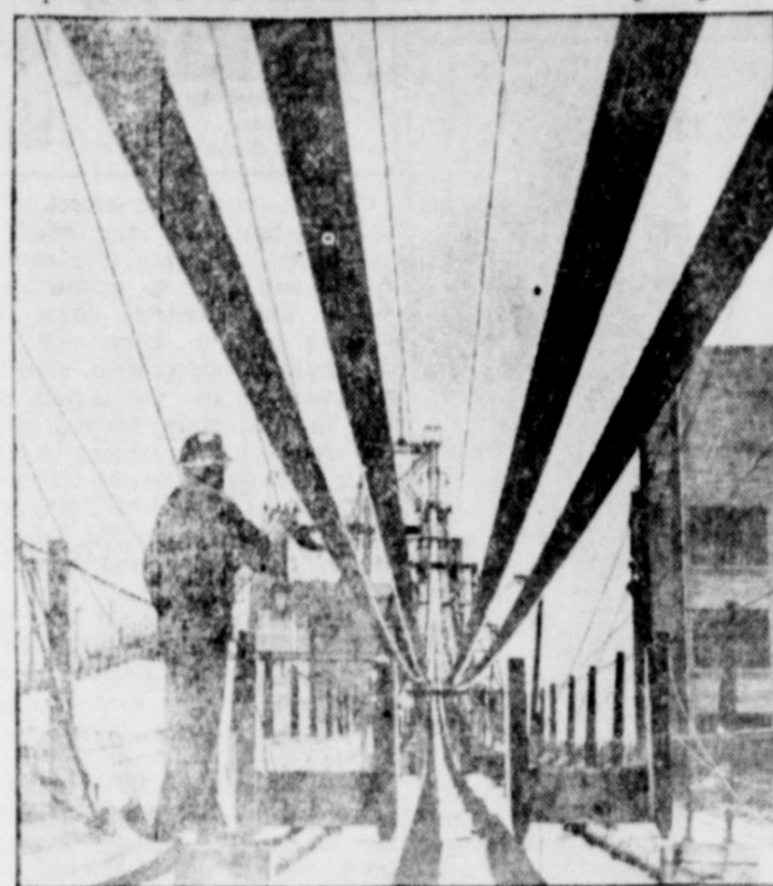
Enough wire to encircle the equator is being spun into the huge cables shown above, which support the giant San Francisco-Oakland Bridge stretching its way across San Francisco Bay. This unique view of the cable-spinning operation was taken from the San Francisco side, looking toward the concrete anchorage of the bridge in the middle of the bay.
