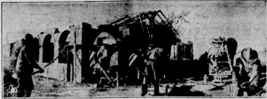
The co-operative effort of the people of Pecos county resulted in the financing of this rock county community house, pictured under construction at Fort Stockton, Texas. The house was planned with the help of the county agent and home demonstration agent, and when completed will be valued at $30,000. It will provide an excellent place for the discussion of farming problems, dinners, games and county canning operations.
