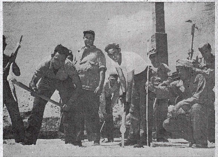
"Taking a reading" here is S-Sgt. J. L. Freeman, one of the construction foremen on the job (at right kneeling). Others in picture are: Pfc. Leo Sperling, Pvt. Martin Eckart, Pvt. Paul Booher, Cpl. Earl Lyons, Cpl. Theodore Lindquist, Pvt. Bill Valdez, S-Sgt. K. W. Hull, and Pfc. Jack Zimmerman.
